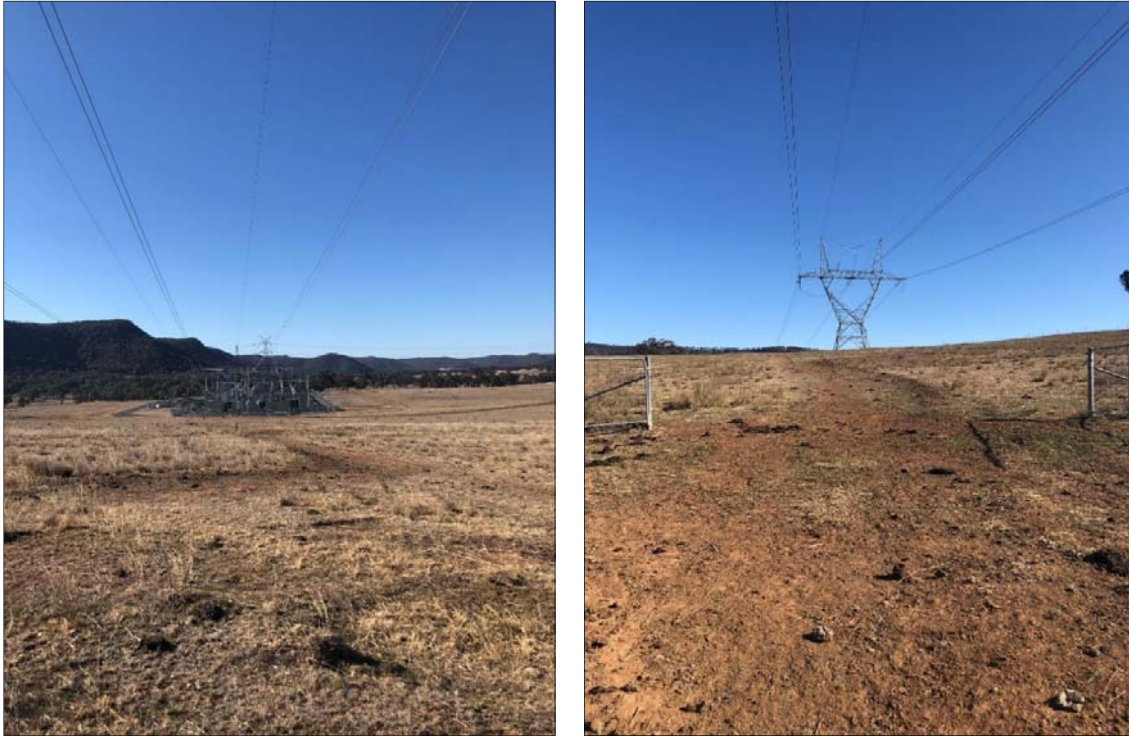
Figure 4-7 330kV transmission line within 60m easement traversing the proposal site and connecting to the Wollar substation.
