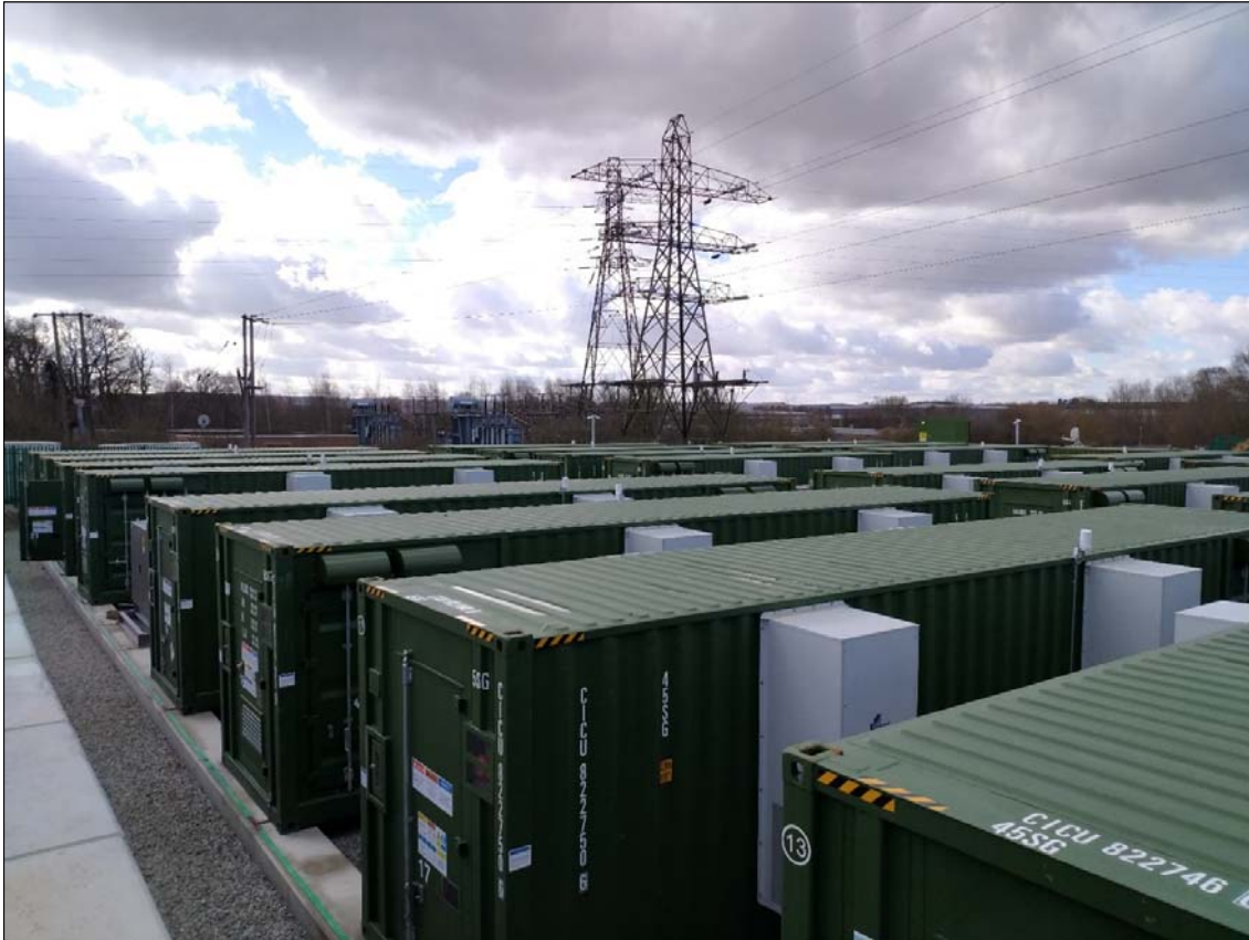
Figure 4-11 Typical battery storage units, located together.
