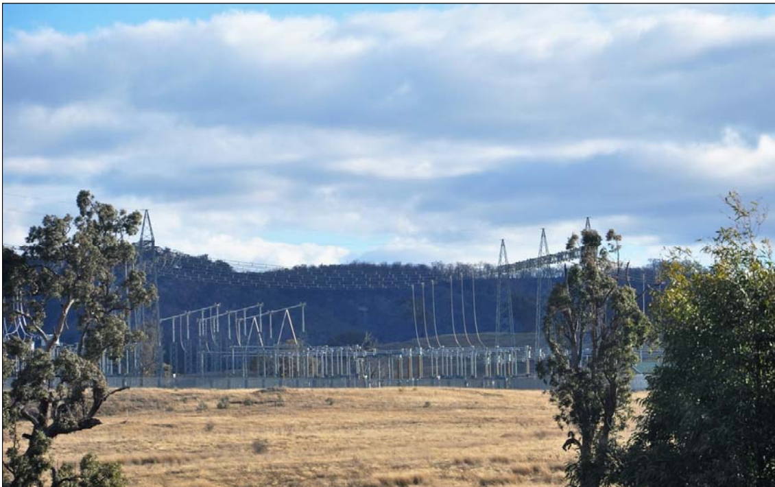
Figure 4-6 Wollar 500/330kV substation.
