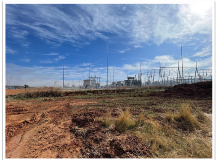
The brand new Transgrid 330KV switchyard, constructed by Downer and ready to receive energy from the solar farm when generating.
