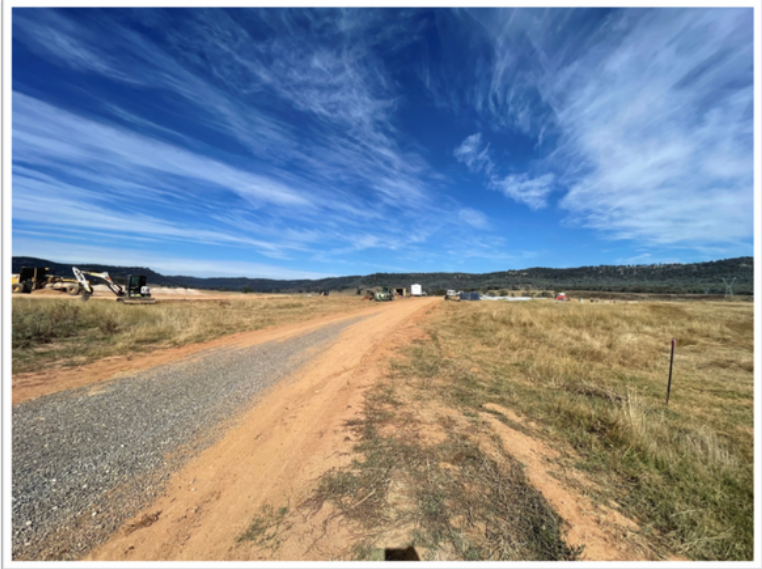
The photo above has captured another beautiful Wollar sky as well as one of our internal project roads mid construction.
