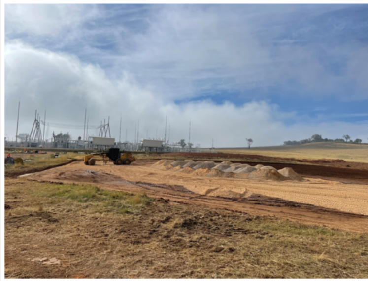
Above shows a grader stockpiling road material that will be distributed around the site as needed. This will help us build internal roads at the Solar Farm allowing safe access for our workers and vehicles.
