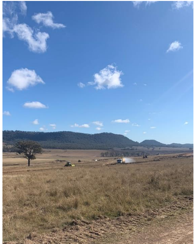
Photo 11: Looking north towards to ST2. Water truck spraying for dust suppression purposes
