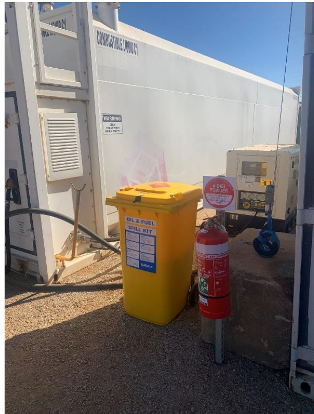
Photo 2: Spill kit in workshop area
