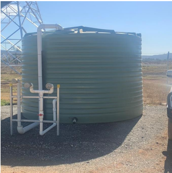
Photo 14: Fire water tank
